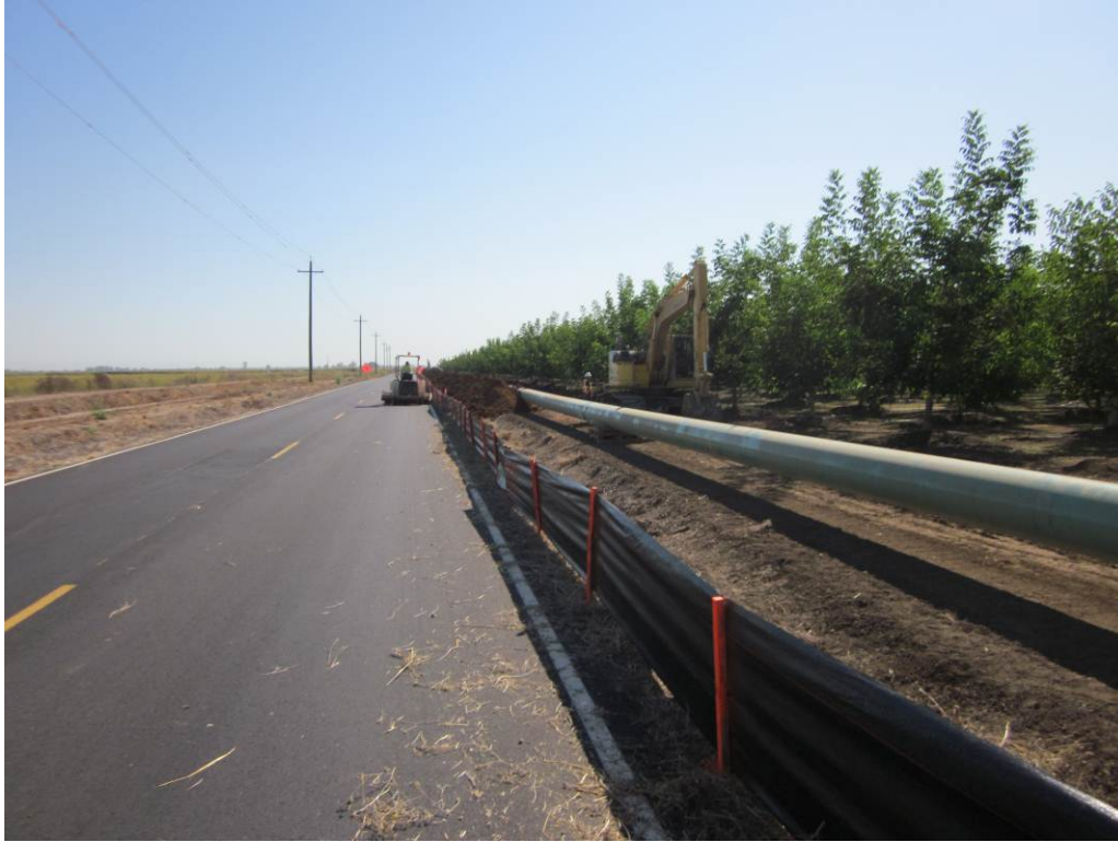
Photo 5: Pipeline staging and trenching along Dirks Road. Street sweeper actively working to remove tracked-out dirt and other project related debris from public roadways.
