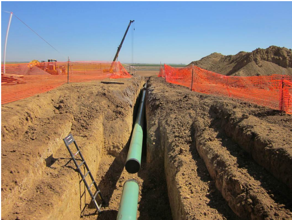
Photo 6: PG&E crews lowering pipe into the trench at the 400-401 line interconnect work area.
